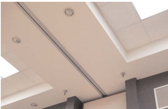
Movable partition system at Multi-purpose
